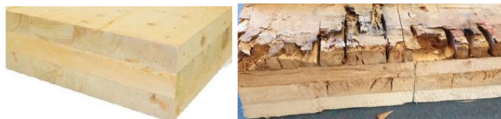
Figure 2. CLT and example of deterioration of CLT flooring under the influence of moisture (Kesik & Martin, 2021)
