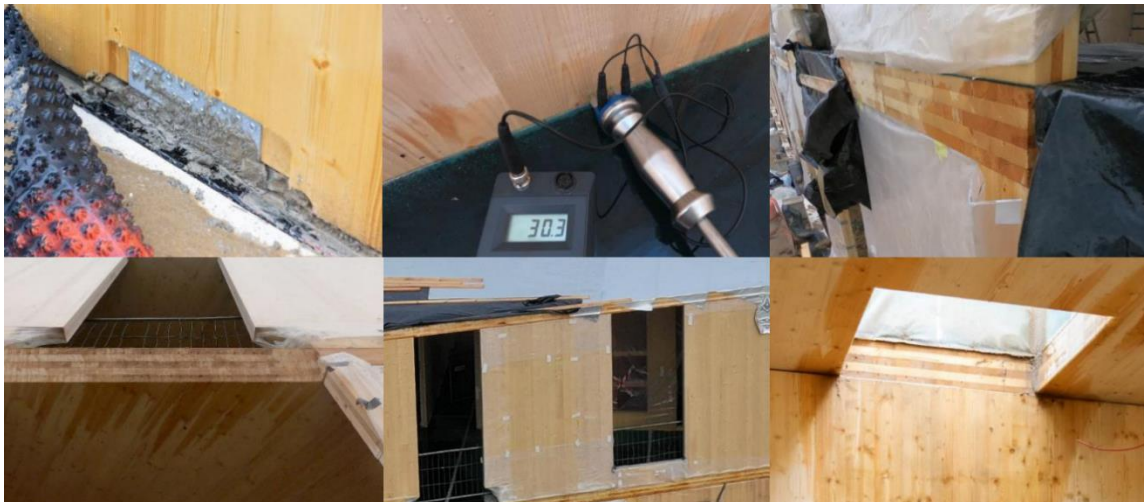
Figure 7. Moisture effects on connections during construction. (Kalbe, Kukk & Kalamees, 2020)
