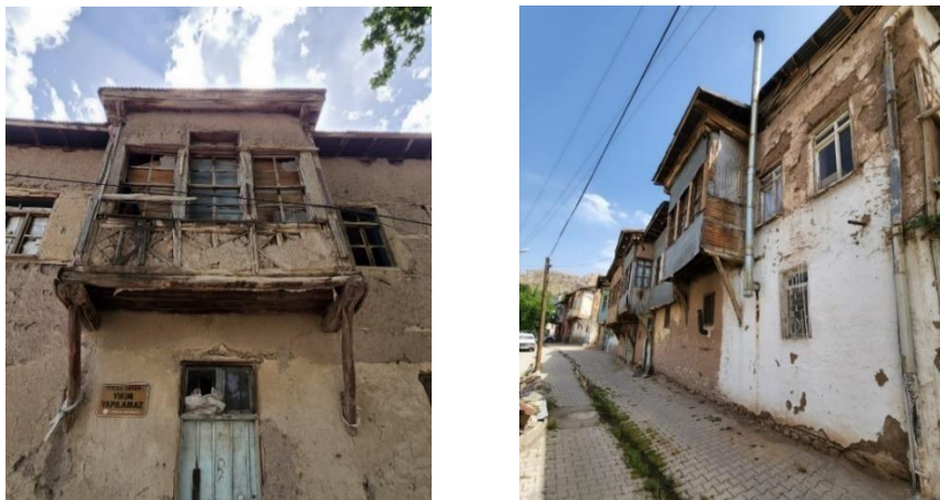
Figure 1. Example of structural problems in walls
