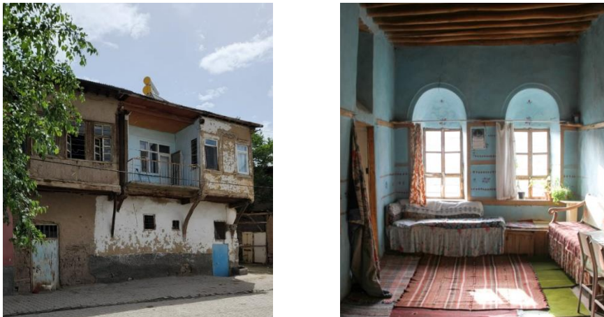
Figure 2. Example of structural problems in joinery
