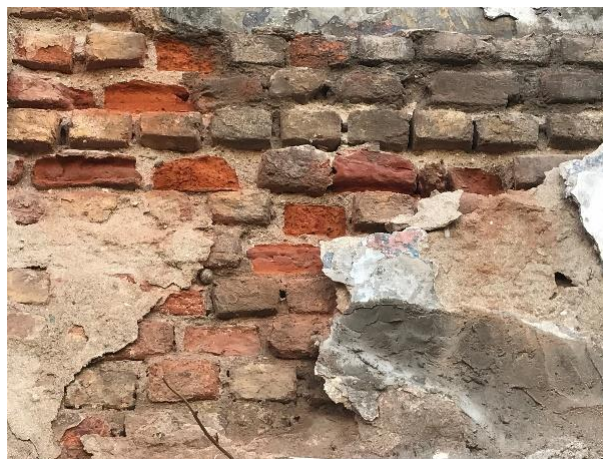
Figure 24. Damage to brickwork caused by the use of strong render (Eryiğit Şenel, 2022)
