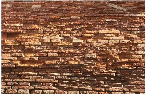
Figure 15. Spalling in frost damaged brick wall (Eryiğit Şenel, 2022)
