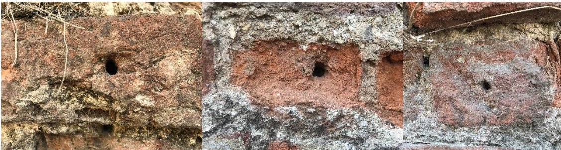
Figure 9. Holes in brick (Eryiğit Şenel, 2022)
