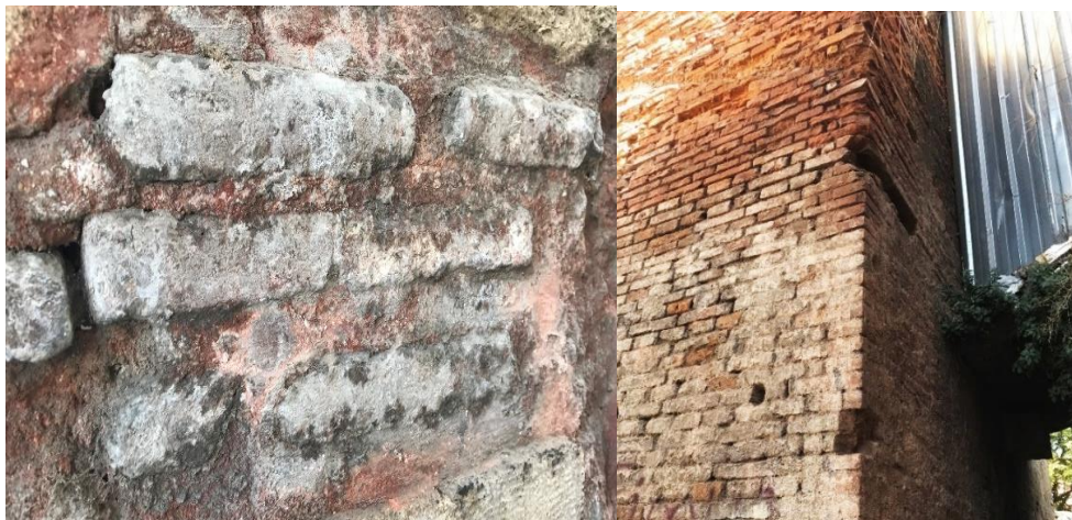
Figure 16. Efflorescence (Eryiğit Şenel, 2022)
