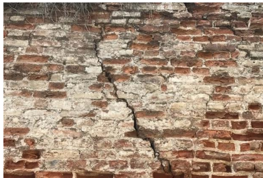
Figure 12. Structural crack in brick wall (Eryiğit Şenel, 2022)
