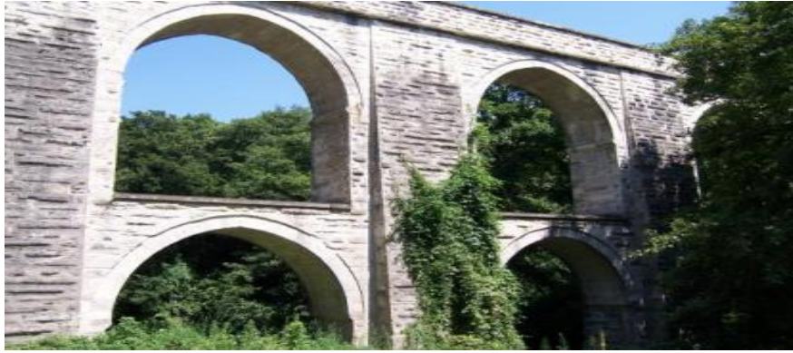
Şekil 6. Paşa Kemerü (Biçkici & Aras, 2013). Historical Aqueducts of İstanbul and Dynamic Analysis of Paşa Kemerü Aqueduct. International. Conference: SE-50EEE, International Conference on Earthquake Engineering)
