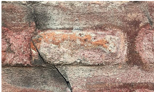
Figure 11. Micro crack (Eryiğit Şenel, 2022)
