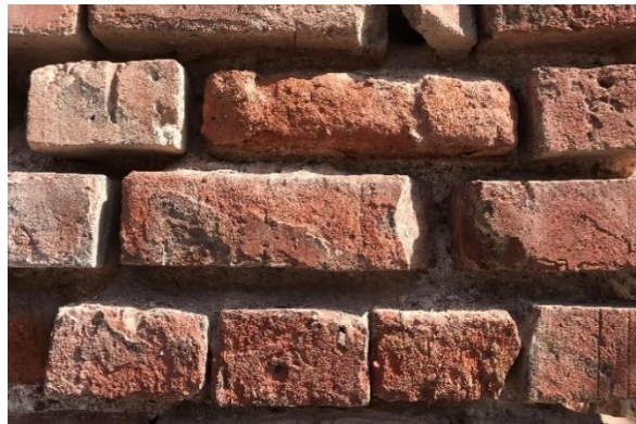
Figure 7. Lack of joints (Eryiğit Şenel, 2022)
