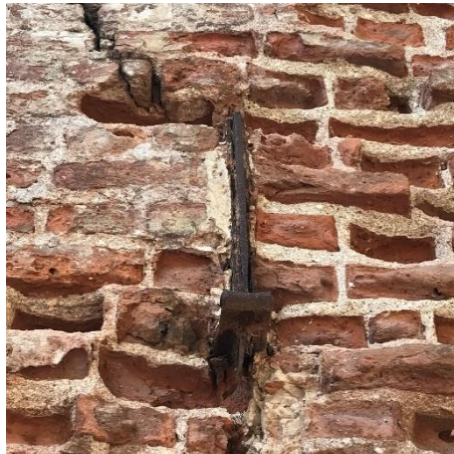
Figure 21. Brick damage caused by the corrosion of iron (Eryiğit Şenel, 2022)
