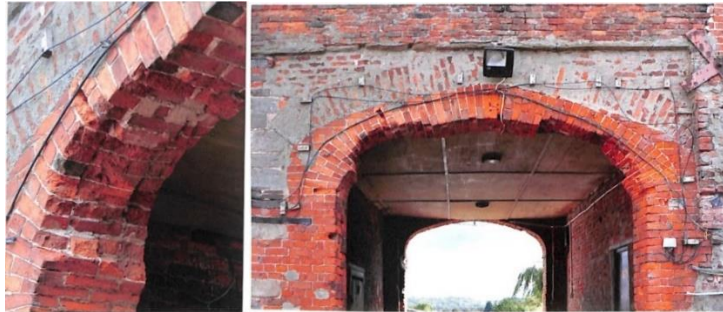
Figure 10. Abrasion of brick arch caused by high vehicles (McCaig, 2015)
