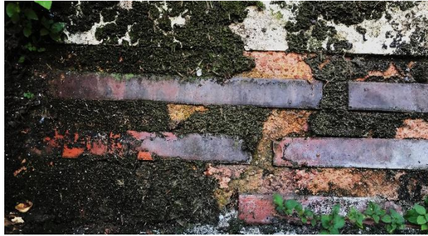
Figure 20. Moss growth on brick wall (Eryiğit Şenel, 2022)
