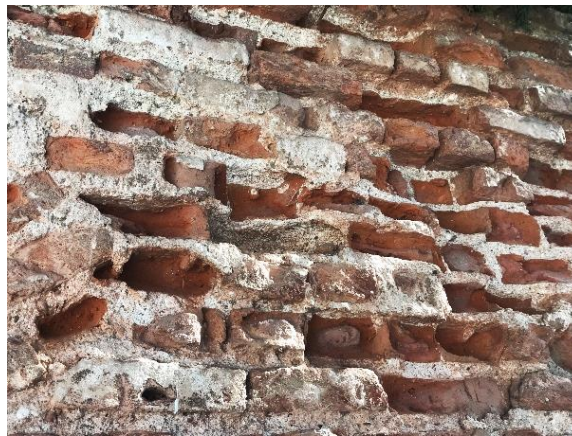
Figure 23. Bricks deteriorated due to the use of dense, impermeable cement mortar (Eryiğit Şenel, 2022)
