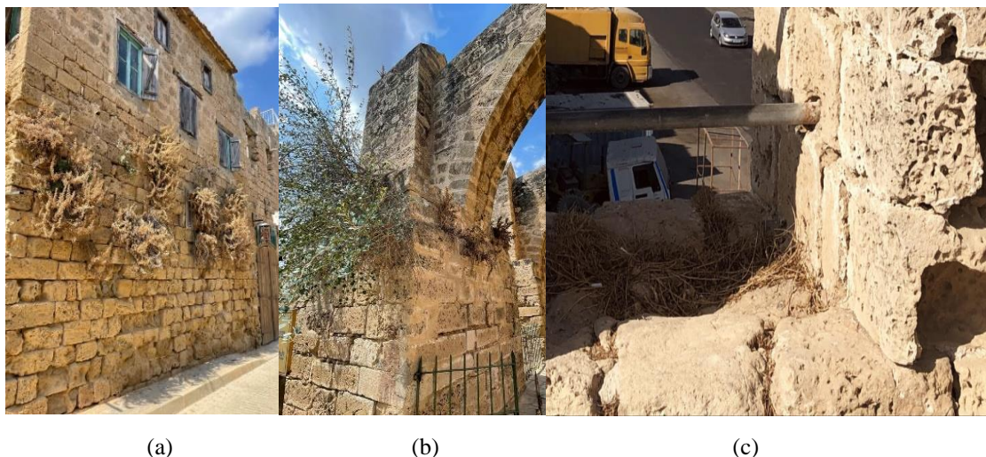
Figure 20. a. Damages caused by plants on the stones of the Old Town Cafe and Bar facade (Öge, 2022), b. Damages caused by plants on the stones of St. Peter and Paul Church (Sinan Pasha Mosque) (Öge, 2022), c. The nesting area formed by the birds causes damage to the castle walls (Öge, 2020).
