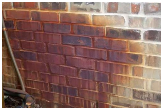
Figure 22. Rust stain (URL 5)
