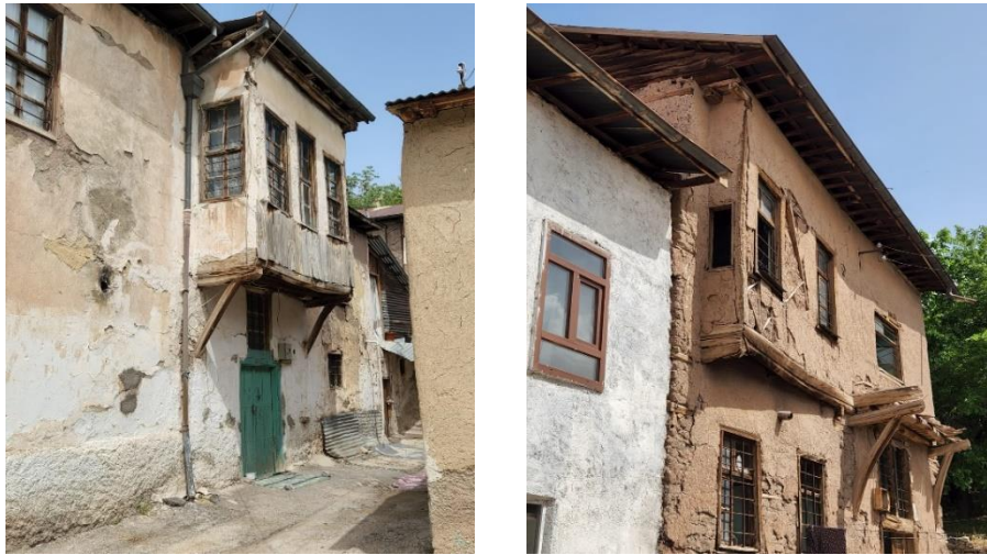
Figure 3. Example of structural problems in joinery
