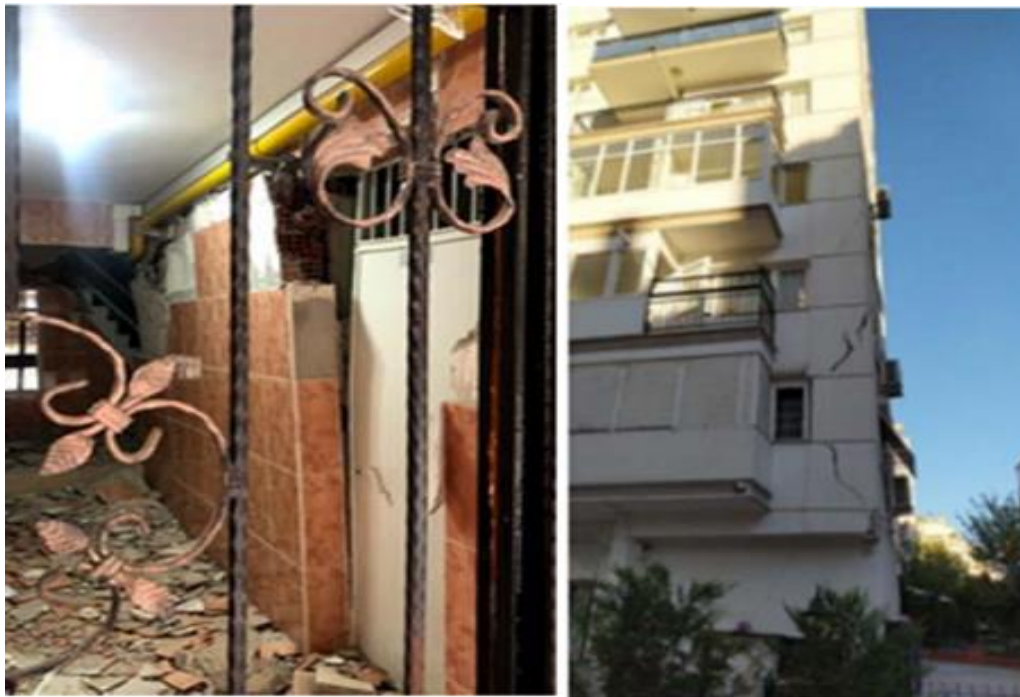
Figure 7. In-plane and out-of-plane infill wall damages (TMMOB, 2020).
